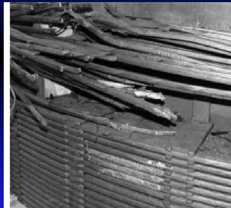
Fig 6: Failure in HV winding of Lethabo #6
