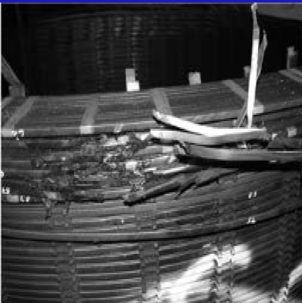
Fig 7: Failure in HV winding of Matimba #4
